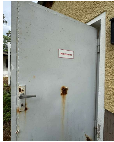
072f Apartmenthaus, Heizraum
